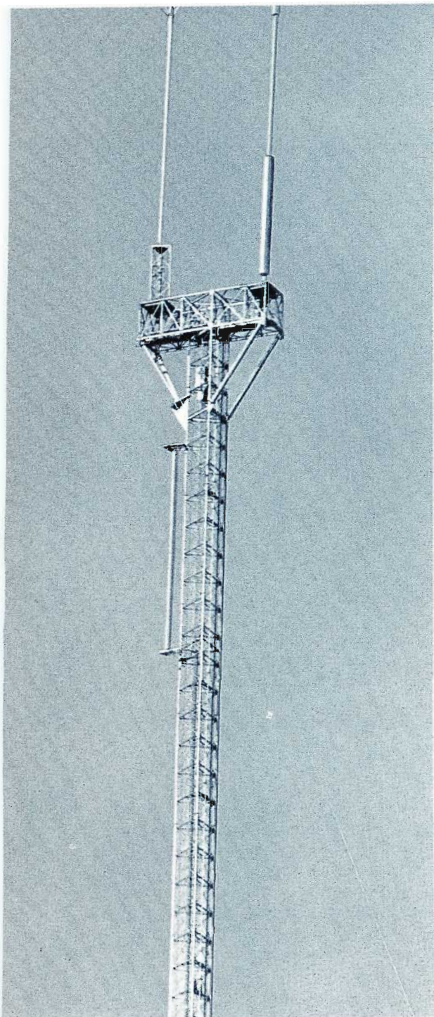
Three-antenna array atop Milwaukee's "T-Bar" tower includes a UHF Type TFU-36JDAS Pylon on left; VHF TW-12A Traveling Wave on right, and Pylon TFU-28DAS side-mounted on tower below the "T".
