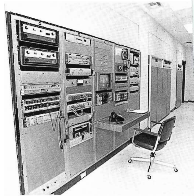
Monitor and control facilities for Ch. 18 and front line cabinets for TTU-55 transmitter are built-in for aesthetics and sound deadening.
