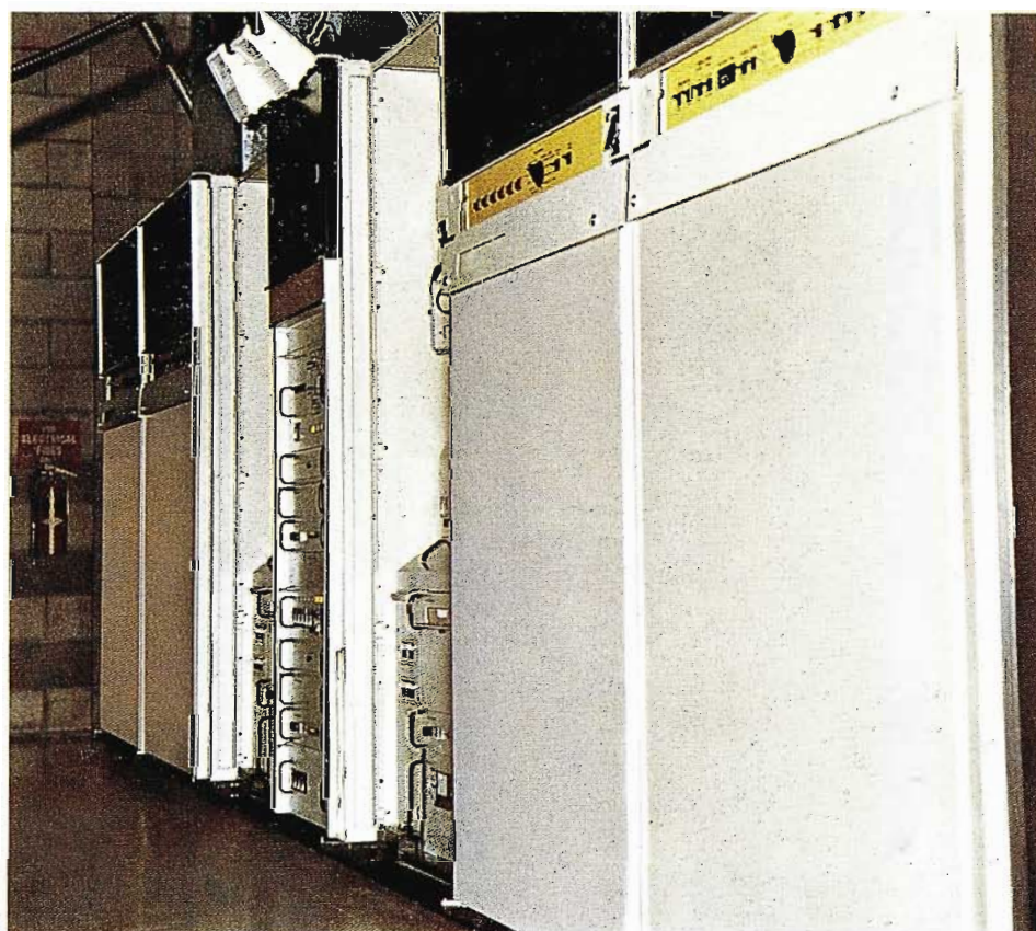
TTG-30/30H Transmitter is a parallel 60 kW system.
